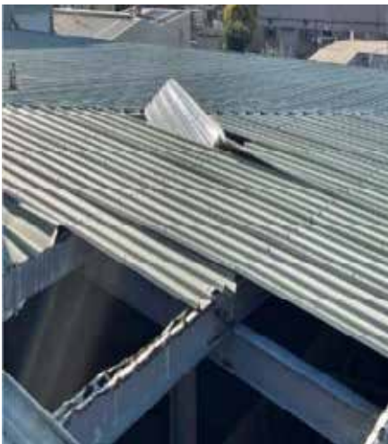
Storm damage October 2021
