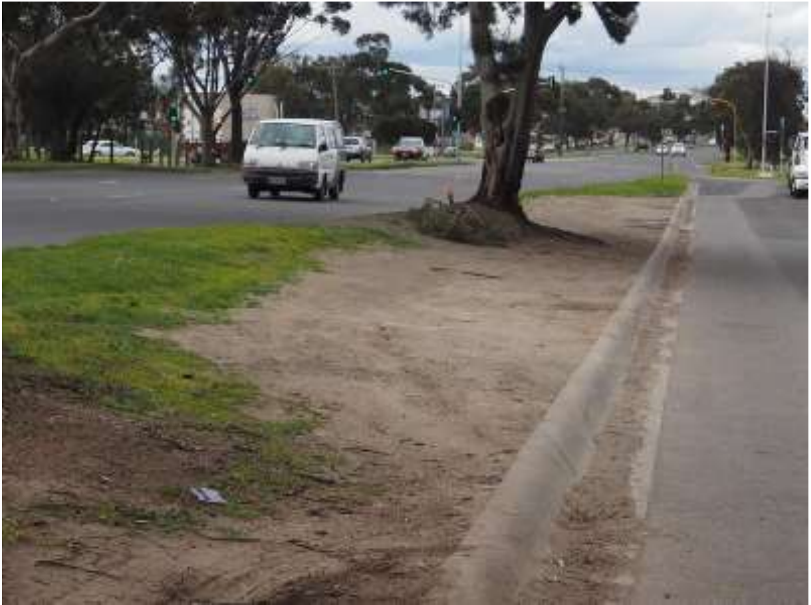
Result of parking on median strip between service Road & Geelong Road!
