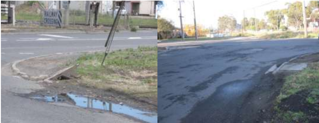
Fig 8 Slides 2 & 3 Dangerous area – before and after
