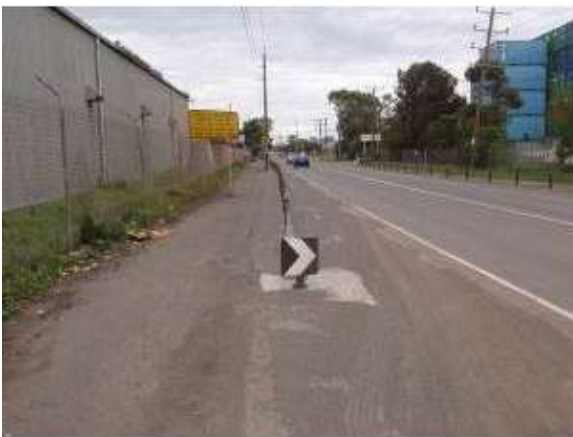
Fig 26 Slides 20 & 21 Francis St, dust visible
